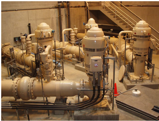
Asset 1: Pumps in station
