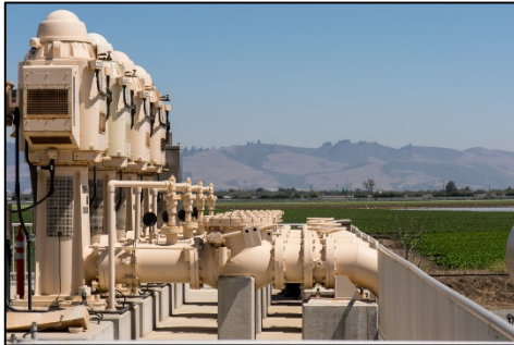
Asset 1: Pumps in station
