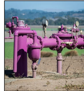
Asset 3: Recycled water pump
