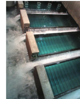
Photo: Chalk Bluff Filter Underdrain System Photo By: Jason Phinney, TMWA Sr. Construction Engineer
