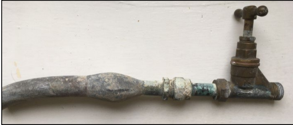
Figure 1. Example of a wip joint connecting a lead pipe to non-lead pipe connector and stop valve. 8
