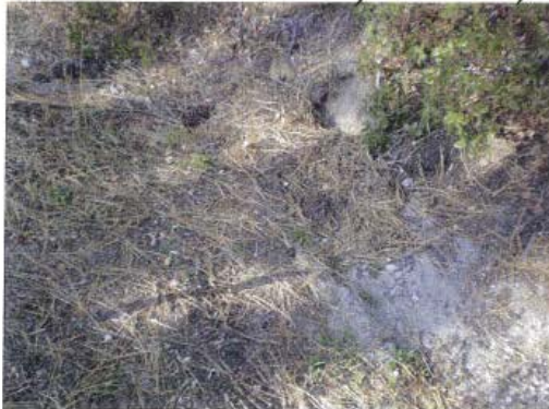
INLET Totally Clogged
