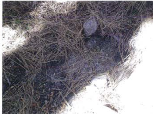
OUTLET (Pipe is Full)
